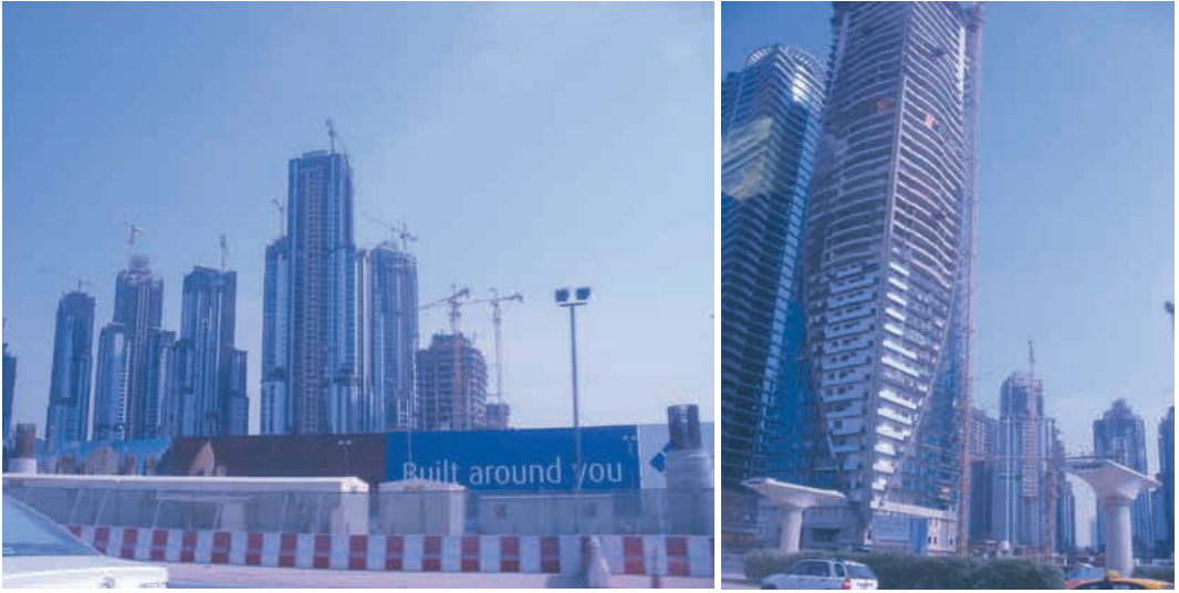
Sheikh Zayed Rd Dubai – the pace of construction in Dubai is phenomenal.
